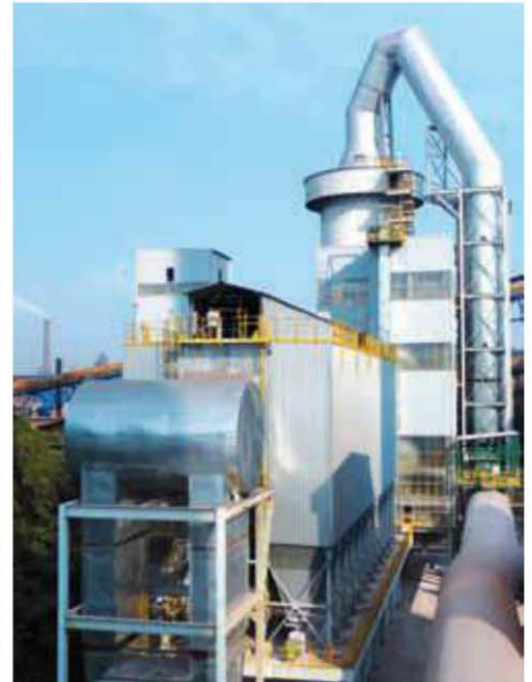
Developed in Europe, exported to Asia: Meros plant in operation at Maanshan Iron & Steel Co.
