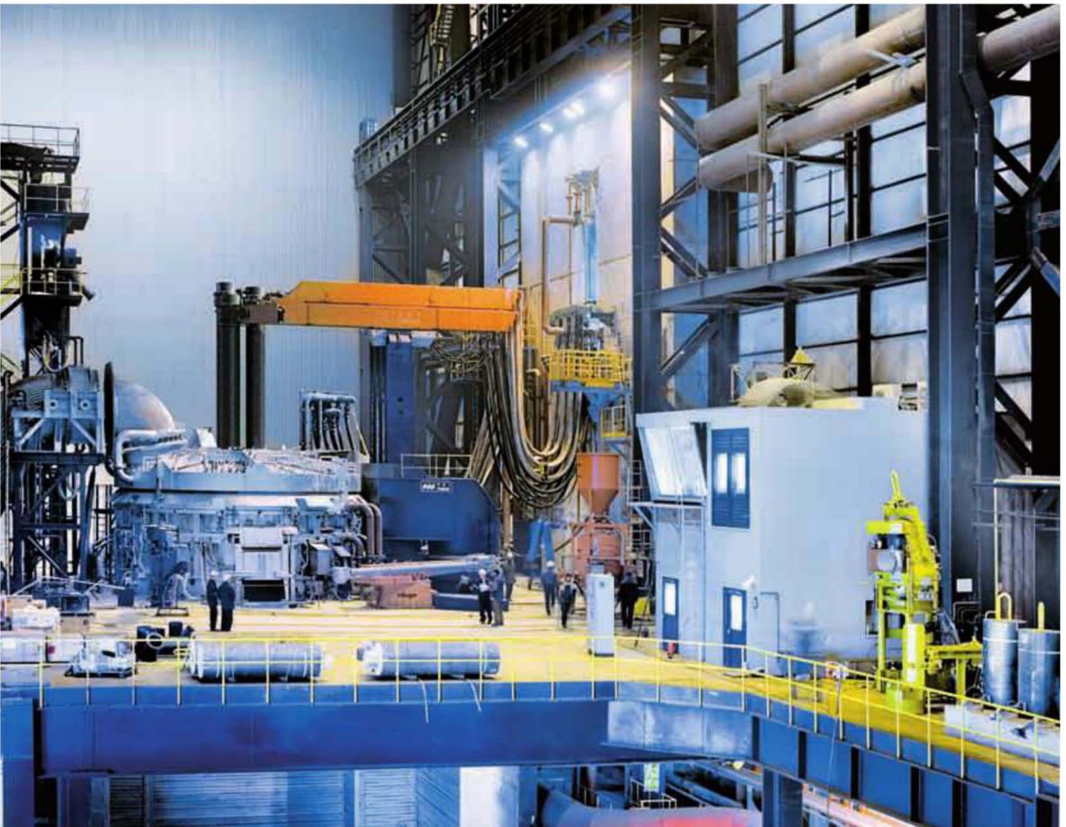
EAF modernization at Çolakoğlu Metalurji A.S., Turkey
