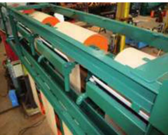
Oil skimmer (left) and the five stands at CSN's No. 3 cold mill
