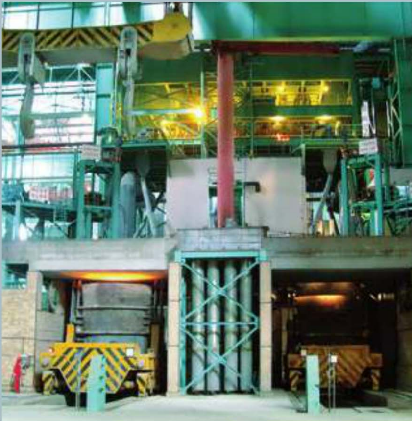
Twin-ladle furnace from Siemens at the Zhangjiagang Hongchang Plate Co. works in China
