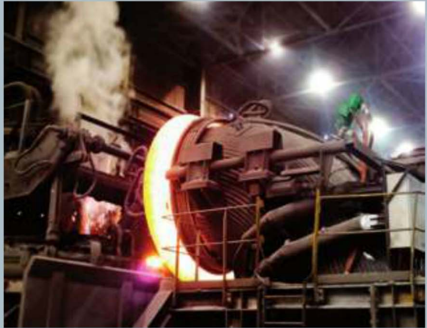
The Lomas offgas monitoring system installed by Siemens along with a holistic process model makes a valuable contribution to lowering costs and increasing operational safety
