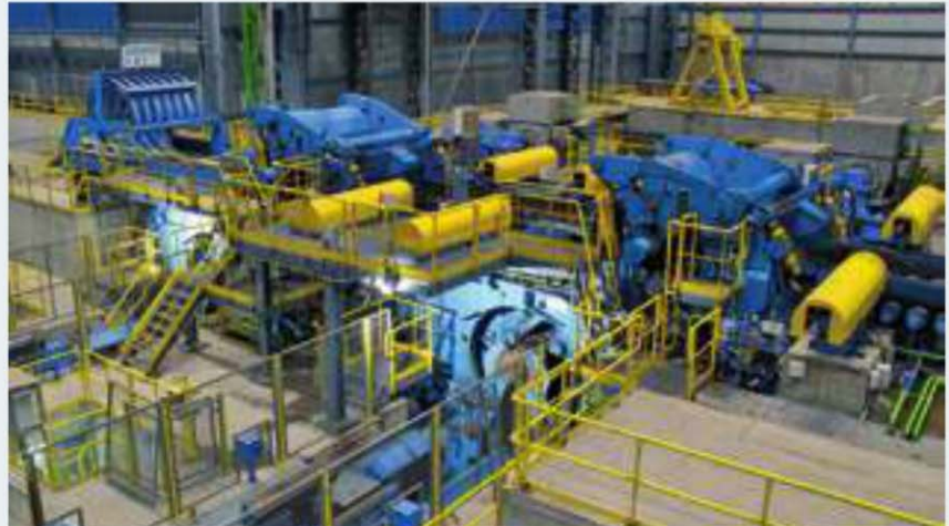
Coiler installed by Siemens at another location but comparable to the one in the hot-rolled strip mill of Tata Steel Europe in IJmuiden, the Netherlands
